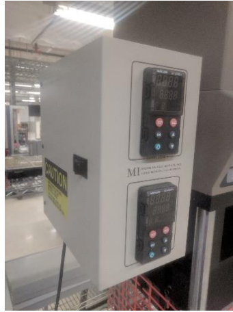
Figure 1 Control Box & Temp Control
